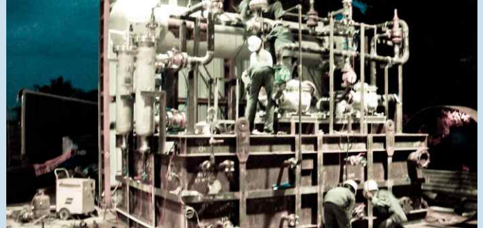
Lube Oil System Under Factory Acceptance Testing (FAT)
