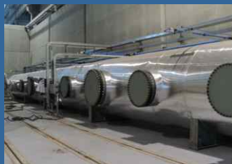
Compressor Discharge plenum
